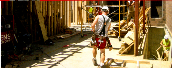
Stevens Construction Corp. crews install a new steel structure inside the façade of an 85-year-old building at 408 W. Gorham St., Madison. The building will soon be home to the Brickhouse BBQ.
