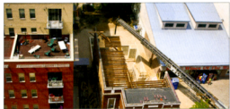
Stevens crews lower a beam into the historic building to create a new floor structure for the retrofitted property. The historic building will retain its 85-year-old façade.
